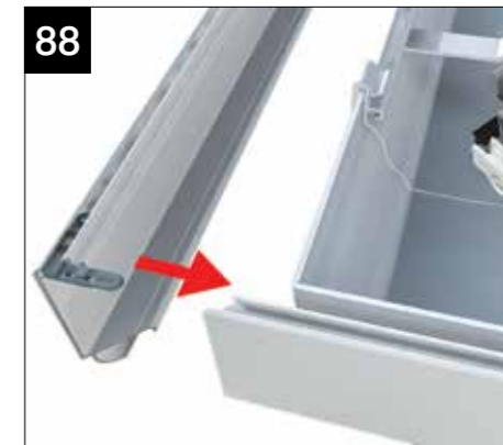
88 Fit cleats as shown earlier for the lower cornice section. Offer up the next middle cornice section. Continue to support lower section as shown in previous step.
