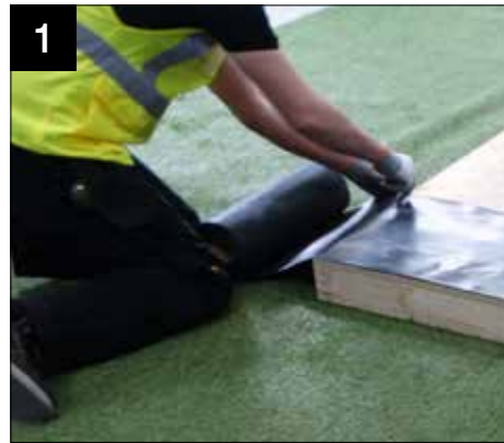
1 Lay out the DPC roll around the perimeter of the base, aligning to the outside edge. Once walls and cills are in place the excess can be trimmed away.
