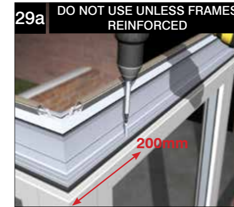
Use 38mm X 4.8mm screws (not supplied) in the position shown. Fix down at 450 centres and within 200mm of each corner. For 60mm frames use the inner eaves extrusion line and outer line of 70mm frames.
