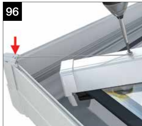
Finally, fix the tie wire using CRN010 screws, to secure the corner.
