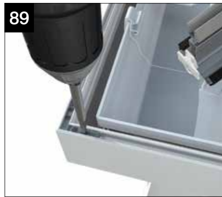
As shown previously it may be advisable to temporarily support the cornice whilst fixing. Secure corners using the cleats (CRN001) and fixings provided (CRN006).
