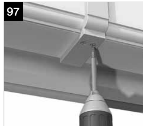
Whilst ensuring that the inline joint remains located in position, screw fix using self drilling screws CRN007
