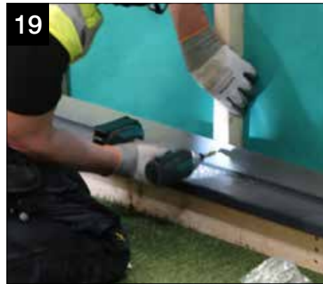
Now secure the top tray and base tray steels to the timber through the pre punched holes using 4.2x25mm wafer head screws provided (NRTF050).
