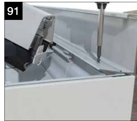
Temporarily support and fit the upper cornice section, using the fixings provided (CRN007).
