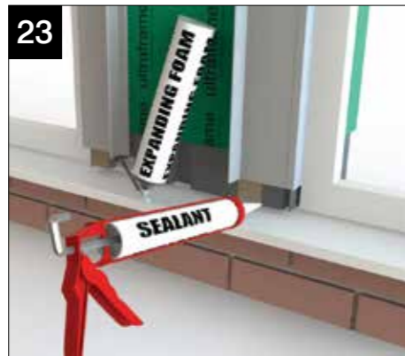
Weatherseal any joints/gaps under columns/walls and between windows/doors/walls and columns. Use foam and/or appropriate sealant.
