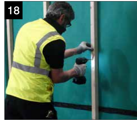
18 Secure the battens to each of the clips by positioning it behind the base tray and top tray steels and centred vertically with the walling panel clips using the provided 5.5mm x 70mm screws (FSW-55-70/10) towards the top and bottom of the timber.
